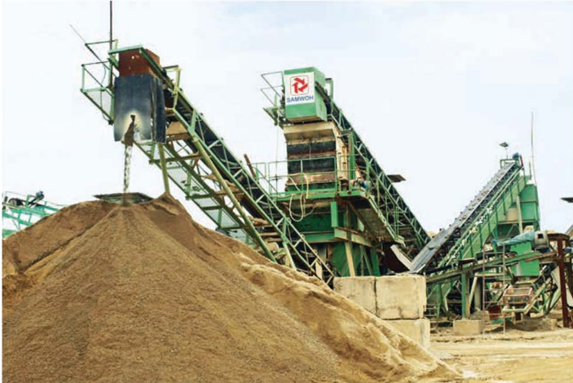
Samwoh's Batching Plant
