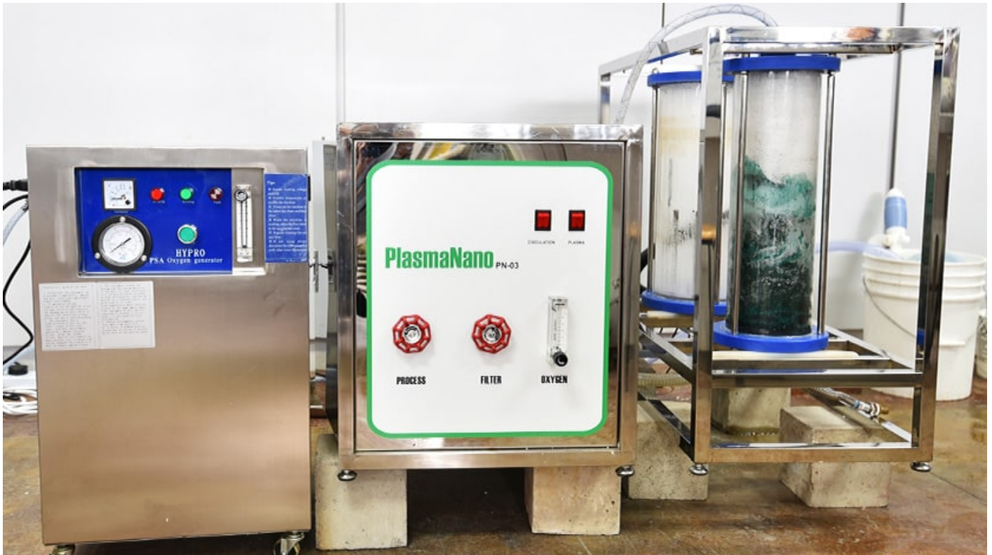
Samwoh’s wastewater treatment plant (Photo credit: Samwoh)
